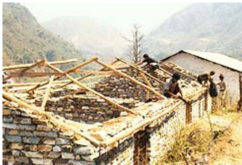
A library being built in Nepal, one of 3,600 schools and libraries Room to Read has helped construct.
